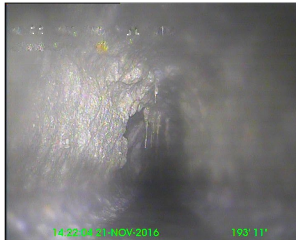
Grease Buildup on sewer pipe
